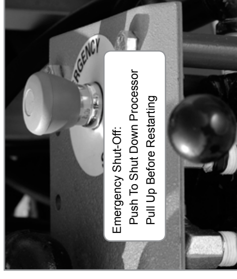
Power Plant Controls – Emergency Shut Off
