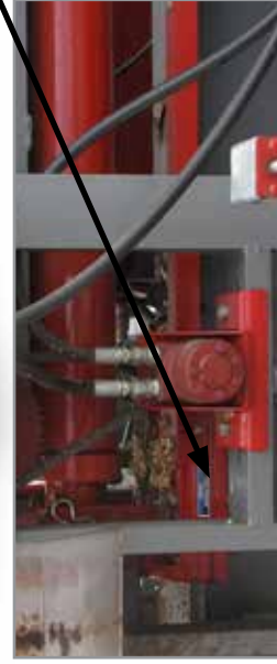
Shown Here: Splitter Cylinder Base
